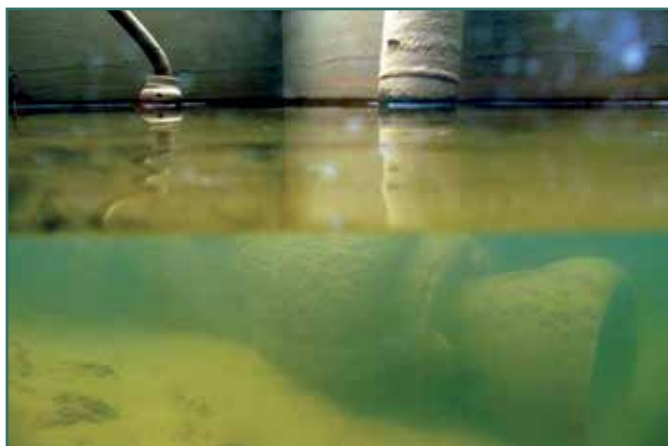
Varkie S55 in process plant sump
